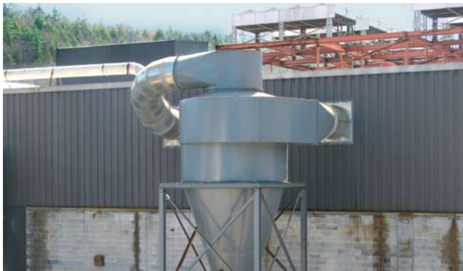
An existing dust collector was retrofitted with a cyclone, powered by a 200 HP Baldor-Reliance Super-E. This unit removes larger particulate and metallic pieces, reducing emissions by 50%.
